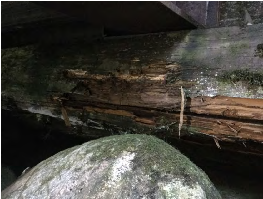
Horizontal crack (4m) on top faced log right bank abutment
